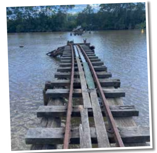
The bridge following the February 2022 flood (Photo: Clive Plater, 8th March 2022)
