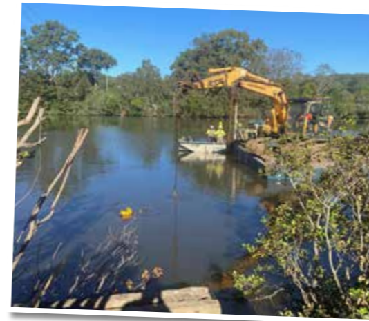
A diver does a final check of the river bed during removal of the bridge. 19th May 2023. (Photo Clive Plater)
