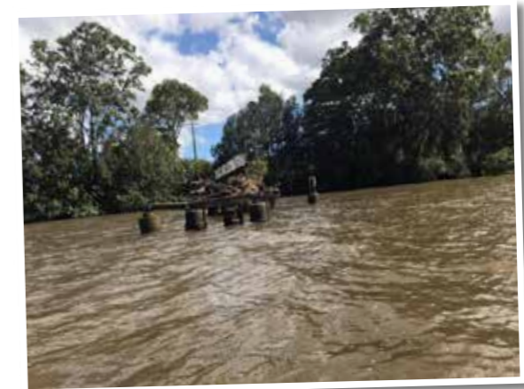
A creeping quick survey on Saturday 5th March, at slack tide of the underwriter structure with 3D scanning sonar shows concrete pillars from the bridge trestle base with trees wedged against the structure under the waterline. The old navigation route is no longer safe and a creeping slow route to the North is currently recommended for vessels.
